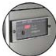
Lesson View Control Panel Cover (Access to Power Only)
